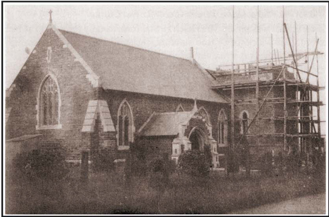
Construction of Christ Church tower c.1910. the nave had been completed in 1904.
